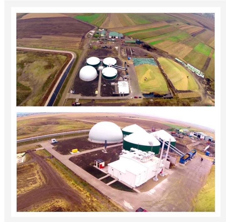
Cogeneration plant Moara: ornicenii Mici, Suceava County
